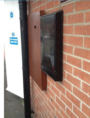
Img009: Electrical Metering
