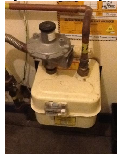
Img012: Gas Meter
