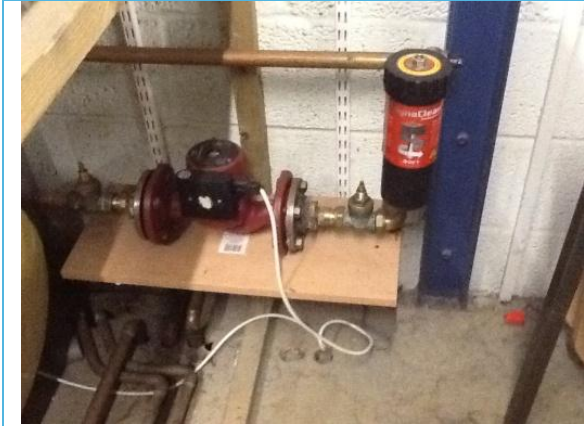
Img007: DHWS Circulating Pump
