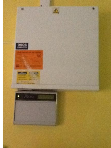
Img014: Intruder Panel
