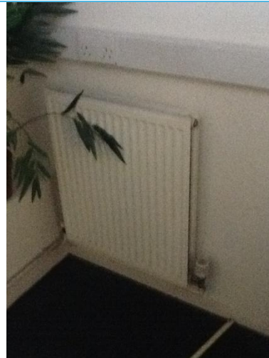
Img020: Typical Radiator
