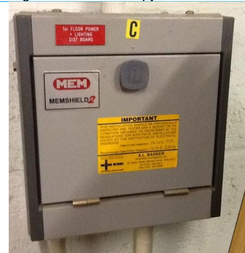
Img018: 1 st Floor Plant Room DB
