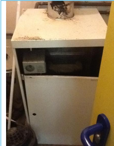
Img019: Primary Boiler
