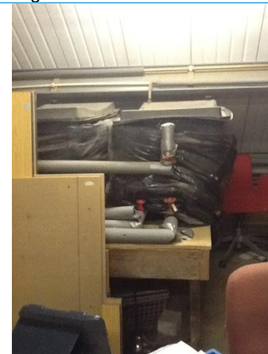
Img006: Water Tanks
